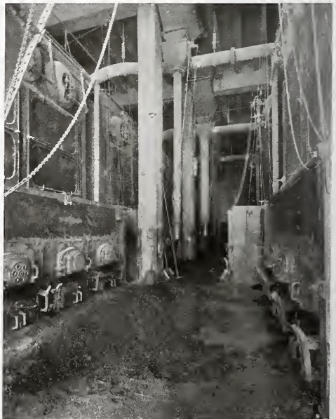
Boiler Room—The Wanamaker Power House, Philadelphia, Pa.
